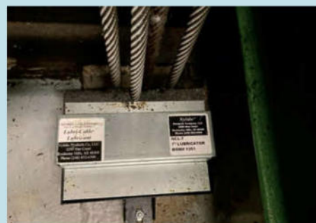
Figure 15: Poor adjustment and positioning of an automatic lubricator causes some ropes not getting lubrication when one rope sits too deeply into the felt and rubs against the metal frame of the device.
