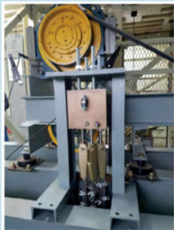
Figure 13: A permanently installed hydraulic rope tension equalizing device
